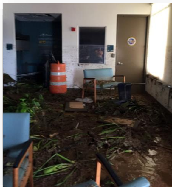
ARECIBO CLINIC DAMAGE - A look at the damage inside the Arecibo VA Community Based Outpatient Clinic in Puerto Rico. The clinic remains closed as Hurricane Maria recovery continues.
